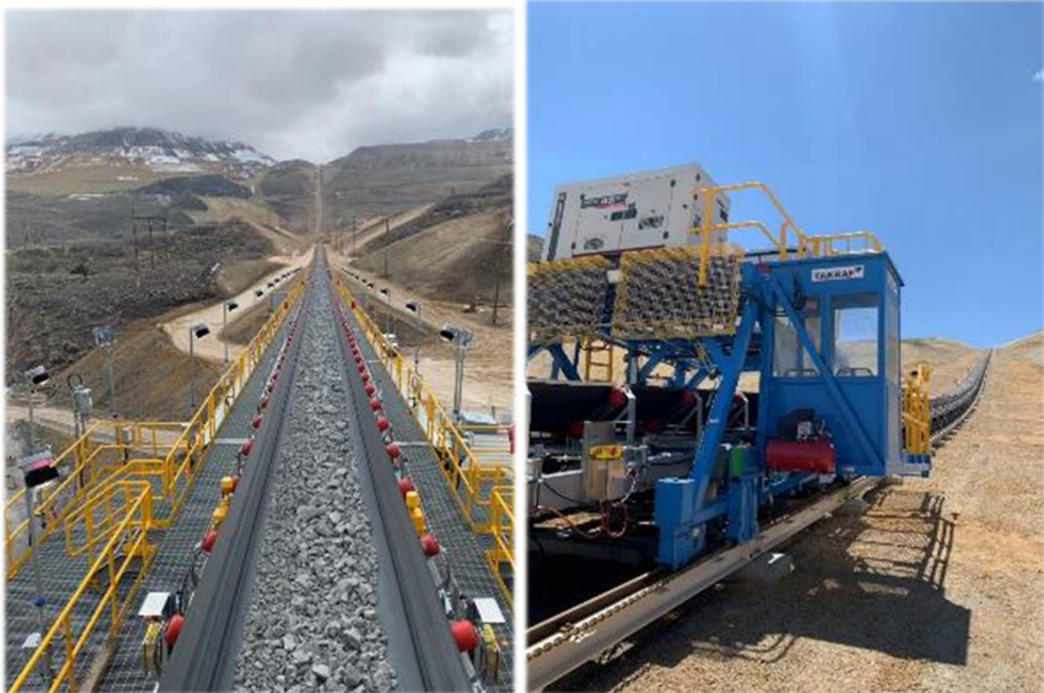
Pic 3 + 4: TAKRAF's US relocation project showing new downhill conveyor managing a 15 degree slope carrying ore to processing facilities on the left and TAKRAF maintenance cart for safe and efficient idler maintenance in position on the right.
